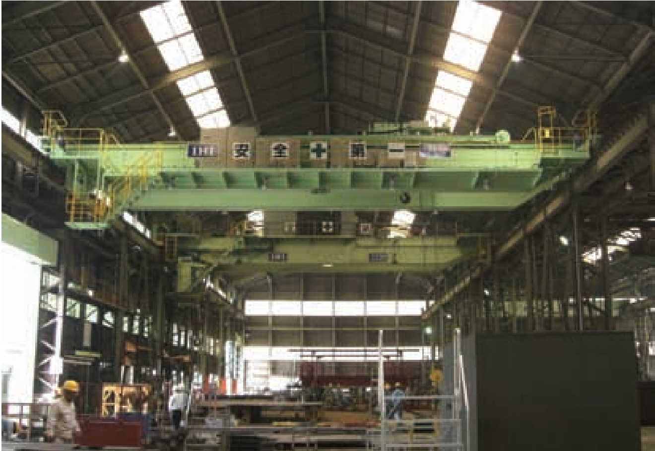
For Machine Shop 30/10t×20m Overhead Traveling Crane
