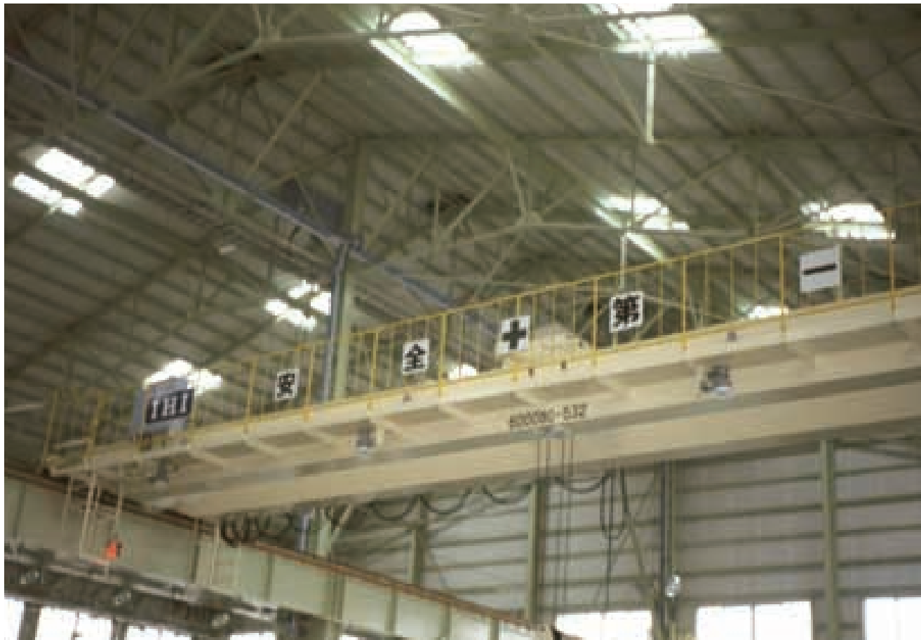
Overhead Traveling Crane with Double Rail Hoist
